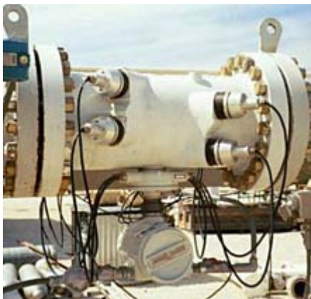
Figure 8. This multipath ultrasonic transit-time flowmeter uses four pairs of transducers to send and receive an ultrasonic signal over the same path length. The values given by the different paths are averaged to obtain gas flow-rate measurements more accurate than those provided by single-path meters. (Photo by Flow Research, courtesy of Emerson Daniel )
