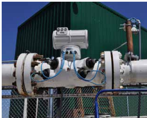
Figure 2. An ultrasonic flowmeter installed in a line at the CEESI flowlab in Colorado.
