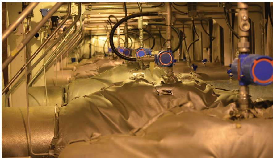
Turbine flowmeters that serve as reference meters for natural gas calibrations at CEESI Iowa.
